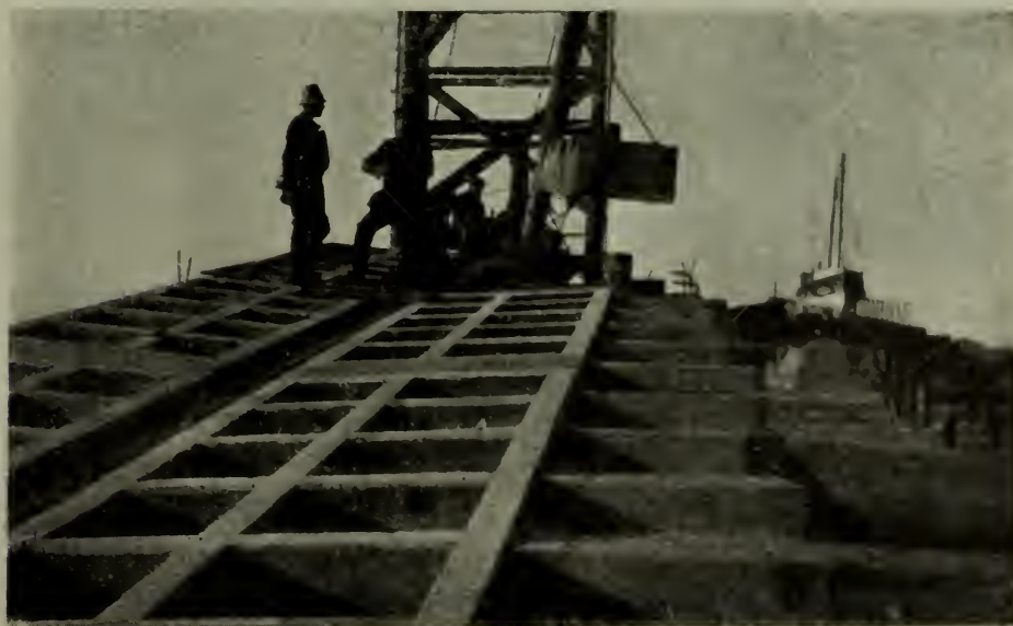
LOOKING UP THE SLIPWAY: STEPPED GANGWAY PANEL BEING PLACED IN POSITION. [This slipway for the lifeboat at Selsey, Sussex, was completed early this year.]
